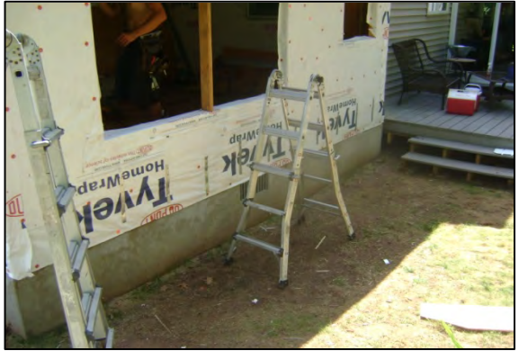
4) During picture , foundation completed and in the process of completing the shell.
